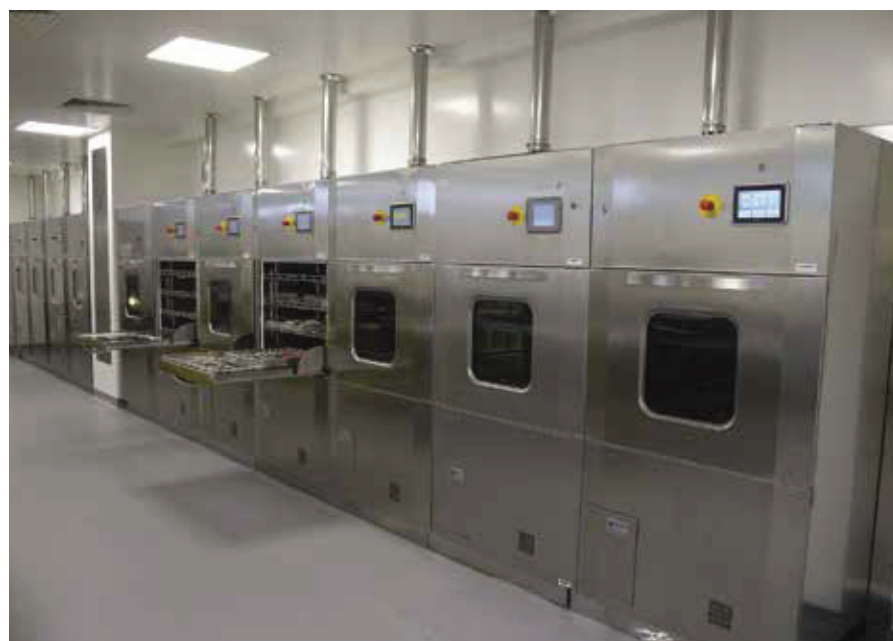
The ten Dekomed DEKO D32 Excel washer-disinfectors. The pass-through hatches can be replaced with further washer-disinfectors for future-proofing
